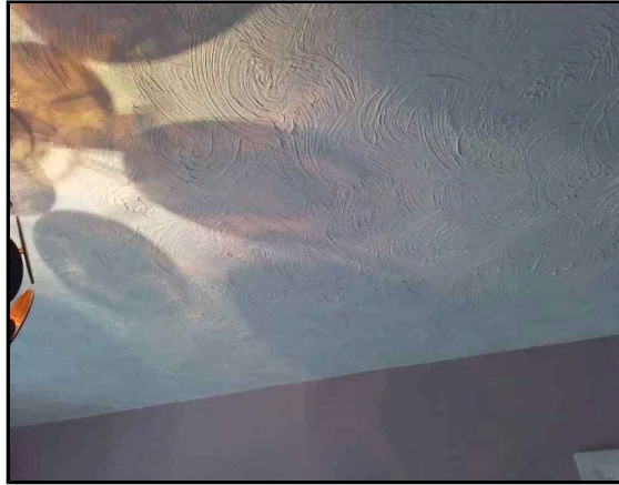
1st Floor Bedroom 4 (1.006) Textured Coating/Paint Ceiling,
