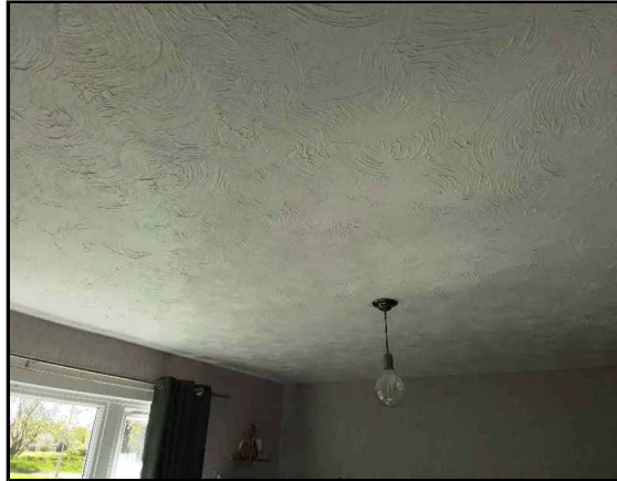
1st Floor Bedroom 1 (1.001) Textured Coating/Paint Ceiling,
