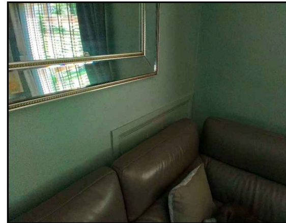
Ground Floor Living Room/Lounge (G.006) Inaccessible Access Panel No access behind access panel
