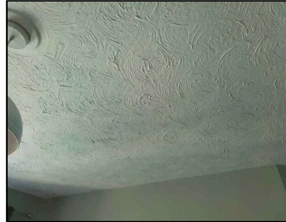
1st Floor Bedroom 2 (1.002) Textured Coating/Paint Ceiling,
