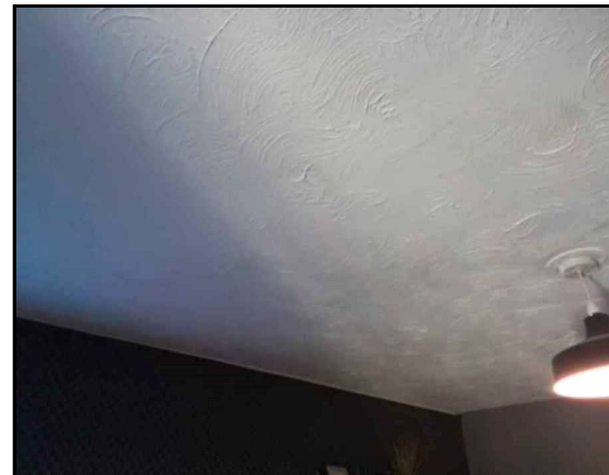
1st Floor Bedroom 3 (1.005) Textured Coating/Paint Ceiling,
