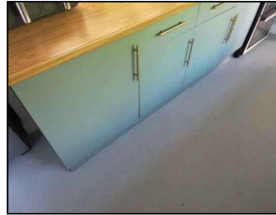
Ground Floor Kitchen (G.003) Inaccessible Boxing No access behind sealed timber kickboards
