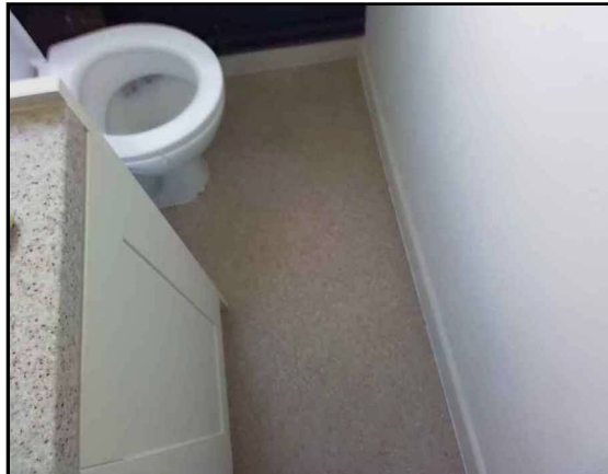
1st Floor Bathroom (1.004) Inaccessible Floor
