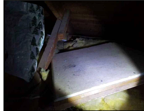
Roof Void Loft Space (R.001) Insulating Board Access Panel/Loft Hatch, Back of hatch
