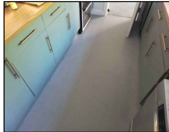
Ground Floor Kitchen (G.003) Inaccessible Floor
