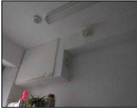
Ground Floor Kitchen (G.006) Inaccessible No access into boxing
