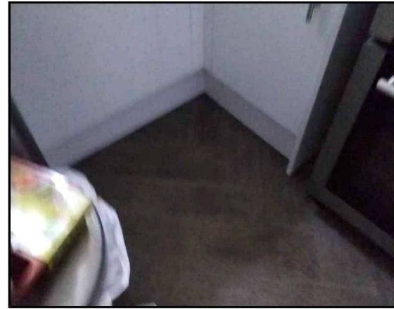
Ground Floor Kitchen (G.006) Inaccessible No access behind kickboards
