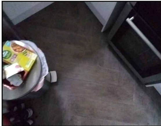
Ground Floor Kitchen (G.006) Inaccessible No access below sealed lino
