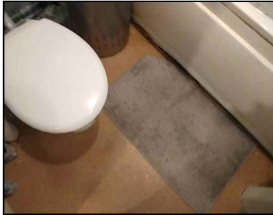
Ground Floor Bathroom (G.002) Inaccessible No access below sealed lino
